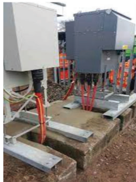
UG Cable termination to equipment
